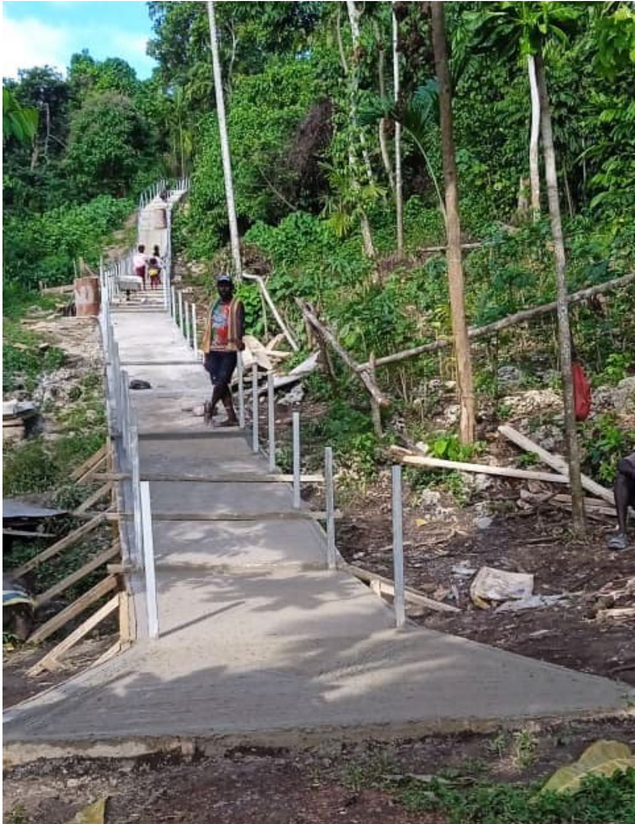
The access road built through the project is the third one in the community of Lemanmanu. It cuts through steep slope and dense vegetation, providing a rapid evacuation way for people living in this area of the coastal community.
