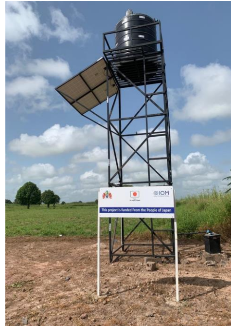
Figure 4 Solar powered borehole in Sabi
