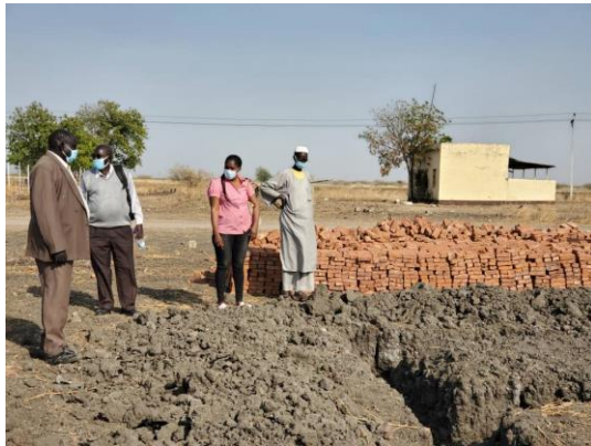
Picture 1: Unfinished infrastructure. Wunthou
